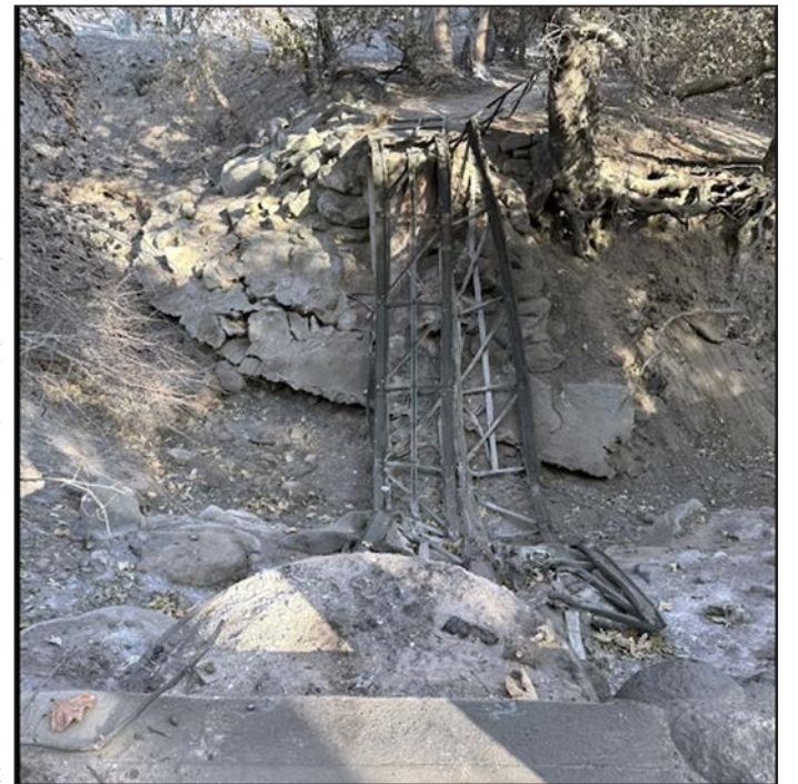
This was the bridge across the stream at Live Oak Park in Bailey Canyon after it burned during the Eaton Fire. A flash flood debris flow during the rains caused it to be washed away completely into the Bailey Canyon Debris Basin.
