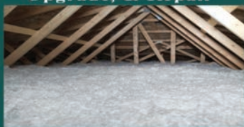
Attic and Wall Insulation
