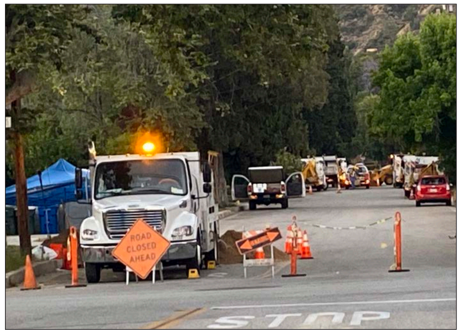
More than 50 workers from Southern California Gas Company will be working around the clock to repair damage. Photo by Maheilia Thomas
