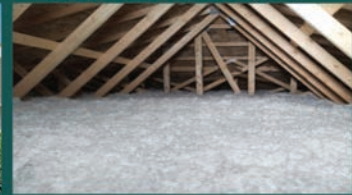
Attic and Wall Insulation
