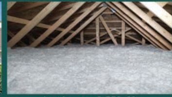
Attic and Wall Insulation
